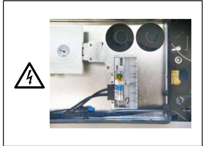
Fig.: Junction box: Danger from electrical voltage
